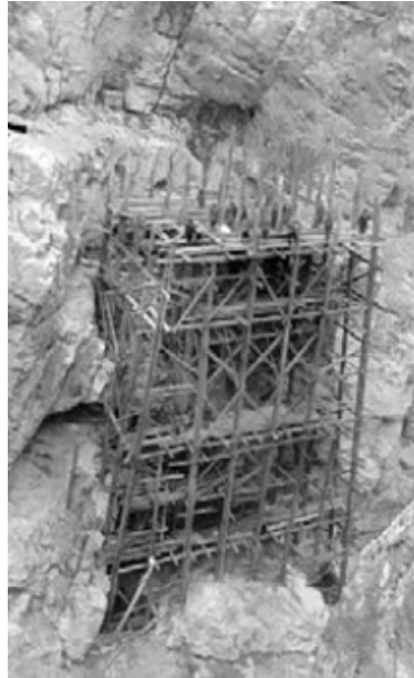
Photo 7: Workers are working on the taller stand of scaffold and increasing its height.
