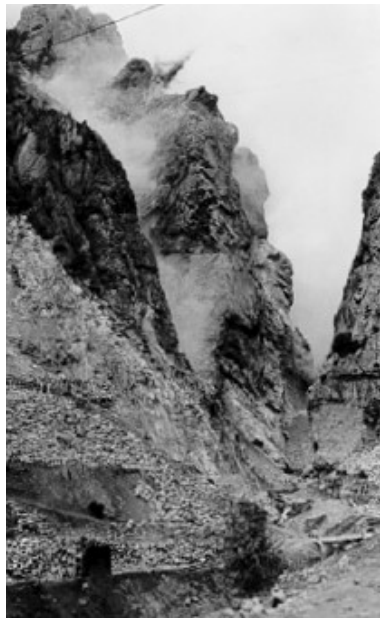
Photo 1: Explosion operation is conducted to provide enough space to install falsework. The cable connected to each side of the valley and used to transfer materials is shown.
