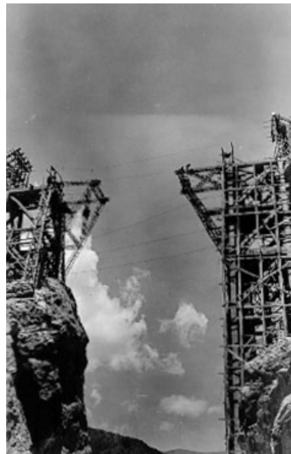
Photo 19: A view of 5 transferring cables
