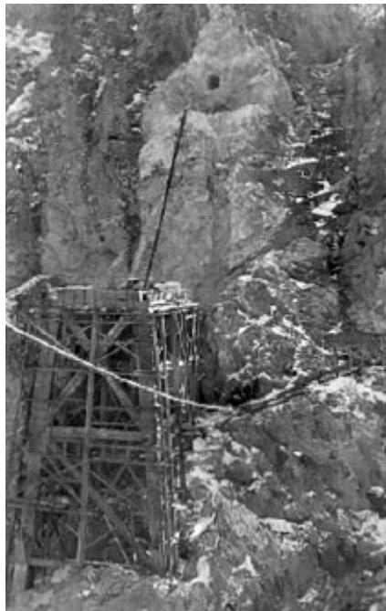
Photo 11: The height of shorter stand is sufficient. The hole on the mountain is the tunnel opening.
