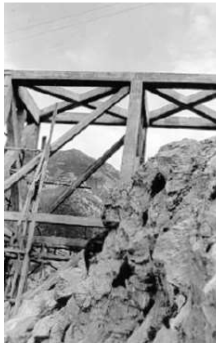
Photo 13: A Closer view of concrete structure that is a constraint for the curved concrete slab
