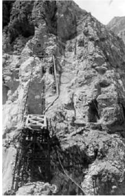
Photo 12: The upper concrete structure is noticeable due to its different color.
