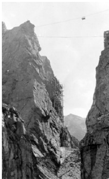
Photo 5: Development of construction operation for the falsework. The concrete structure is built in the falsework.
