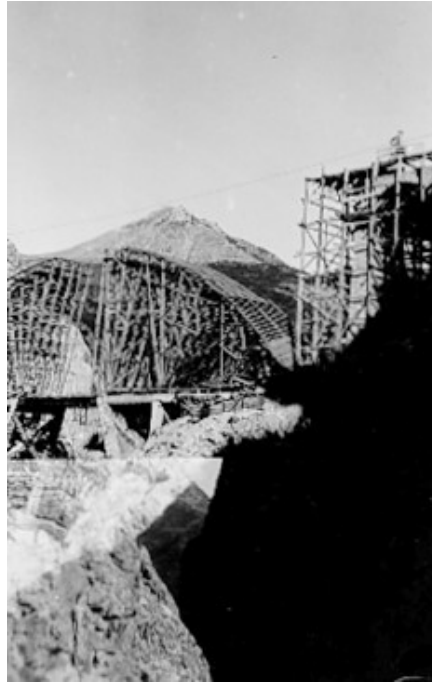
Photo 24: A view of two parts of a curved slab and the opening and ending of the tunnel
